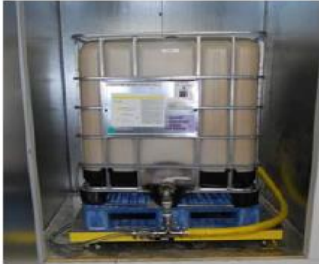
Liquid Yeast dosing & Storage
